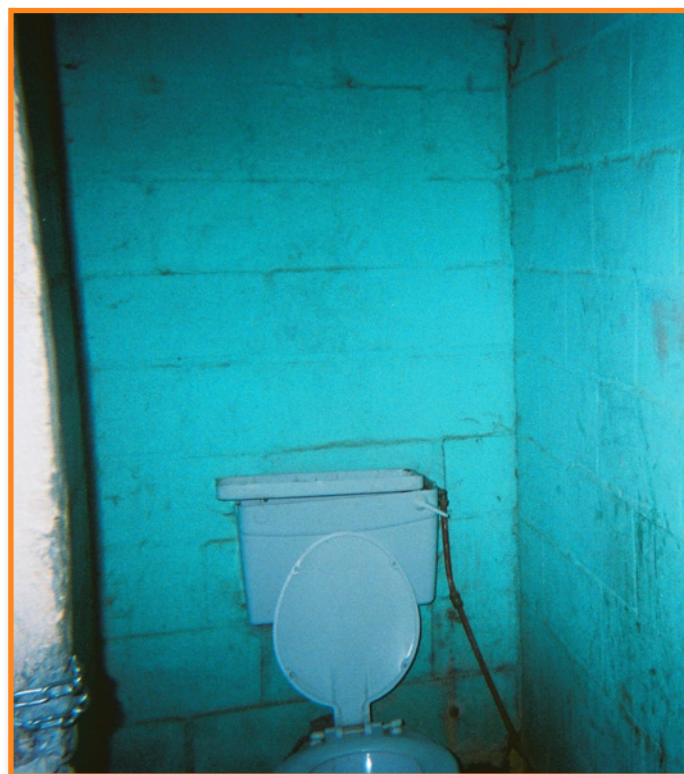
“This is our toilet. It is far from home and is used by 15 houses. I want people to see it.” — Caption by the potographer, a Stellenbosch learner.
